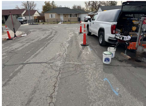
Photograph 2: Pavement Condition at C-24-07
