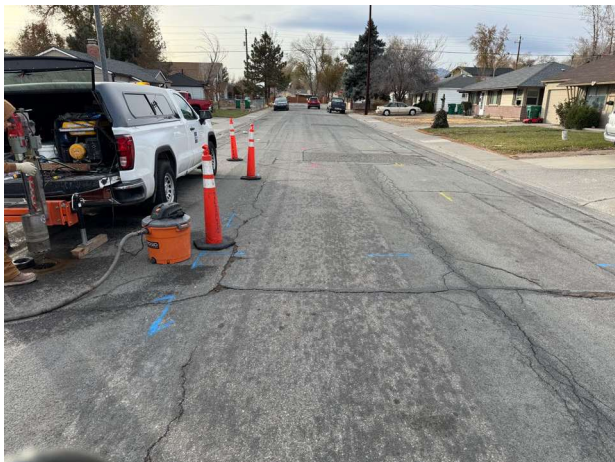
Photograph 3: Pavement Condition at C-24-08
