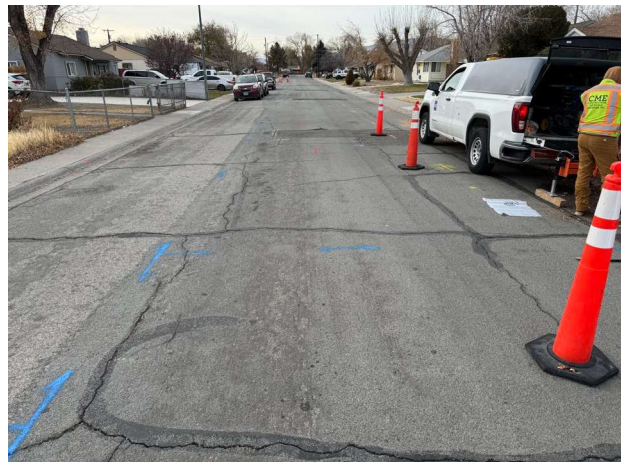
Photograph 4: Pavement Condition at C-24-09
