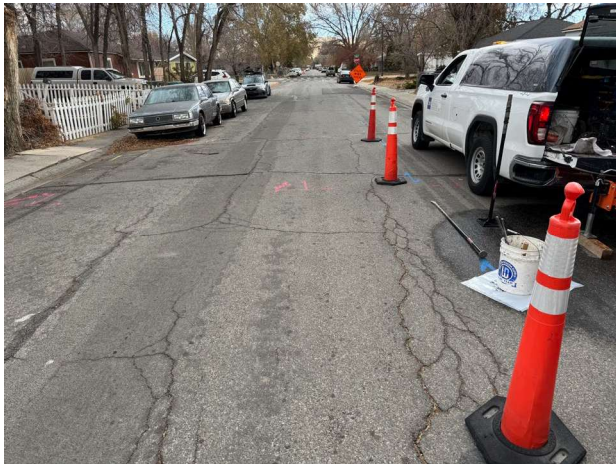
Photograph 7: Pavement Condition at C-24-12
