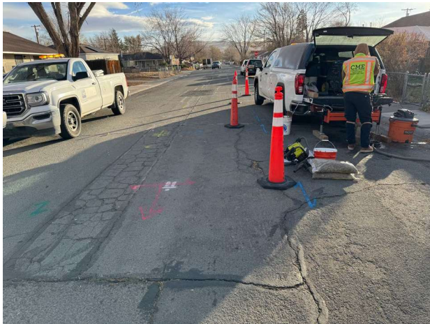
Photograph 5: Pavement Condition at C-24-10
