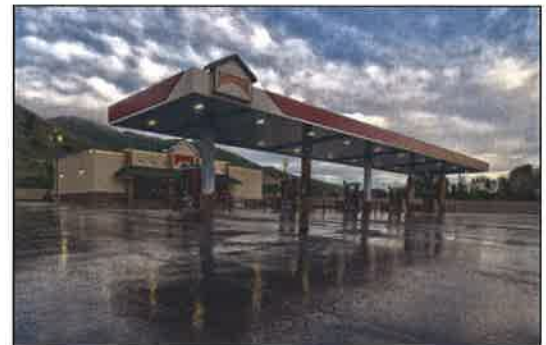
2.5.17 (g) Canopies consistent in material and color with the main building are important.
