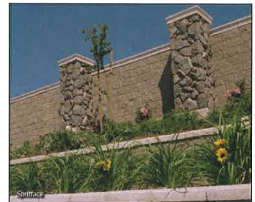
2.5.10 (f) Solid walls incorporating pilasters and landscaping break up the monotony of a large expansive wall.
