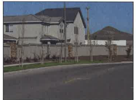
2.4.8 (d)(e) Perimeter fencing adjacent to streets with pilasters and complimentary materials provide for an attractive project statement.
