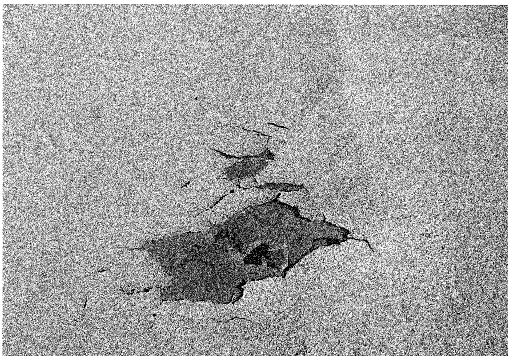
Photo 6: Typical damaged area in polyurethane foam insulation on top of cover. Area shown is approximately 1 foot square. About 25 such areas exist.
