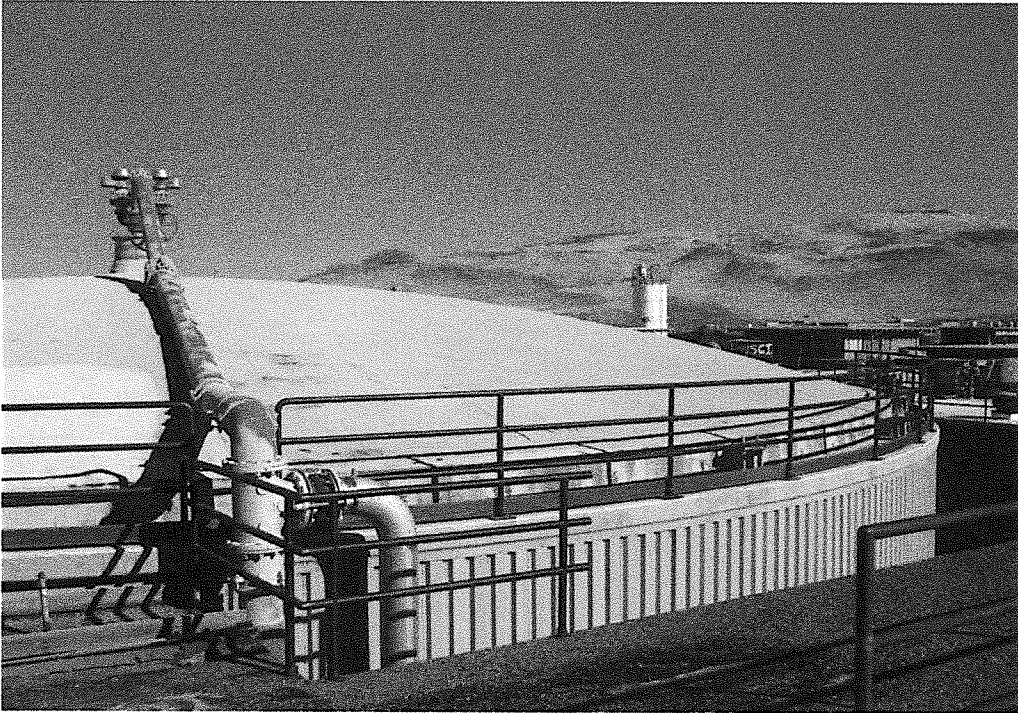
Photo 1: Overview of digester cover. Gray surface is coated polyurethane foam insulation. Edge of steel cover is visible behind handrail. Two cover connection brackets are visible at photo right center.
