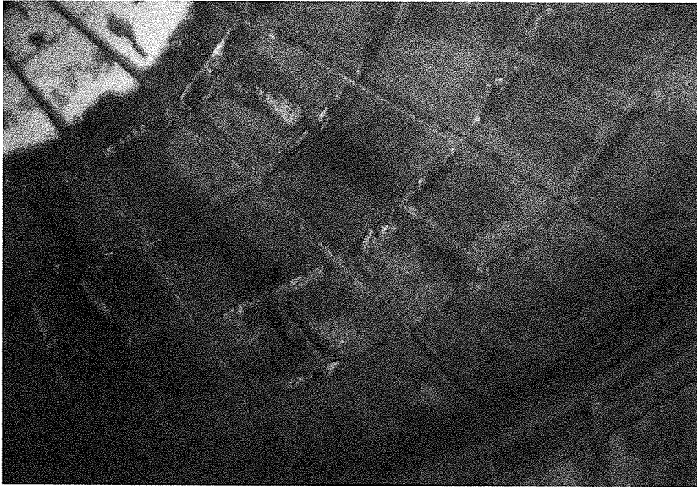
Photo 3: Typical condition of cover interior. Center of cover is at photo upper left. Black areas appear to be coated with coal tar epoxy. Orange areas are rusty steel exposed at areas of deteriorated coating.
