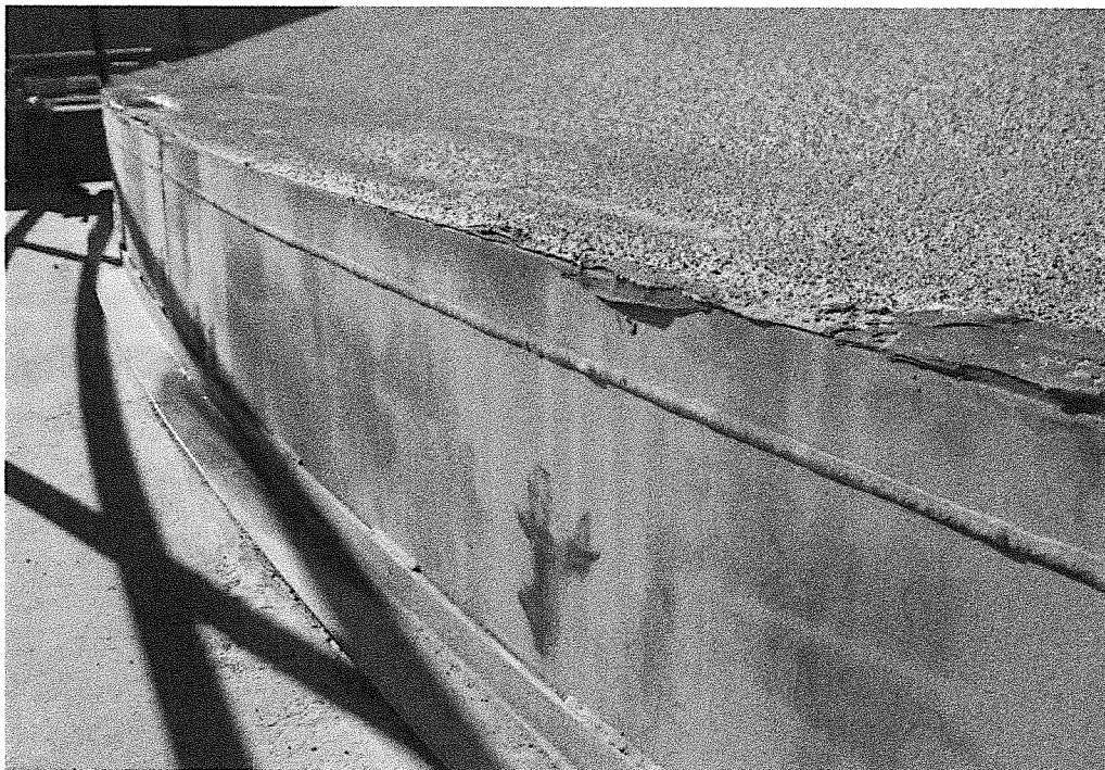
Photo 2: Skirt' area of cover. Top of concrete tank wall is at photo lower left. Cover includes coated foam insulation, sidewall, and steel angle. Connection bracket is visible at far top left of photo.
