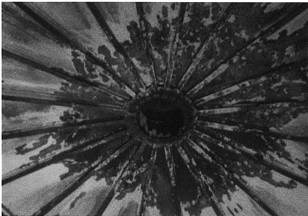
Photo 5: Center portion of cover as viewed from floor of digester. White areas are deposits from digester operation. Orange-brown areas are rusted steel, including connection bolts at center ring.
