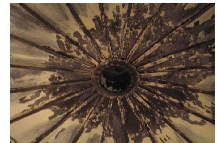
Photo 5: Center portion of cover as viewed from floor of digester. White areas are deposits from digester operation. Orange-brown areas are rusted steel, including connection bolts at center ring.
