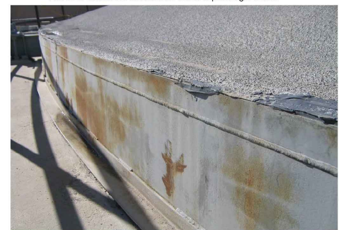
Photo 2: Skirt area of cover. Top of concrete tank wall is at photo lower left. Cover includes coated foam insulation, sidewall, and steel angle. Connection bracket is visible at far top left of photo.
