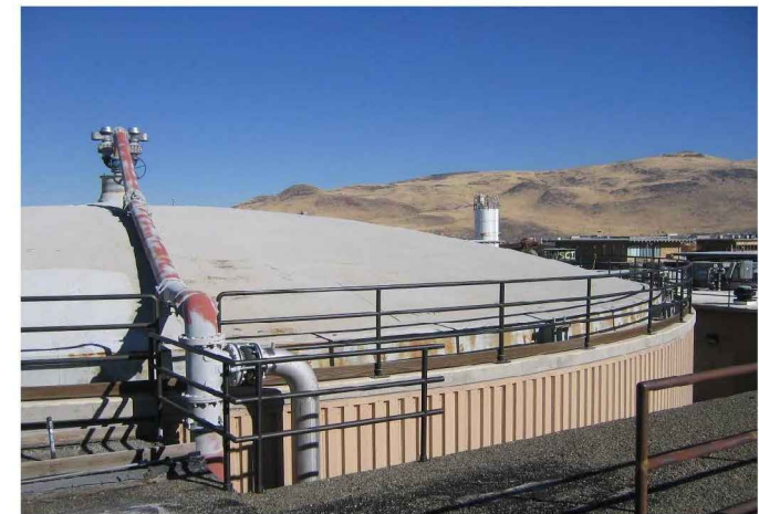
Photo 1: Overview of digester cover. Gray surface is coated polyurethane foam insulation. Edge of steel cover is visible behind handrail. Two cover connection brackets are visible at photo right center.
