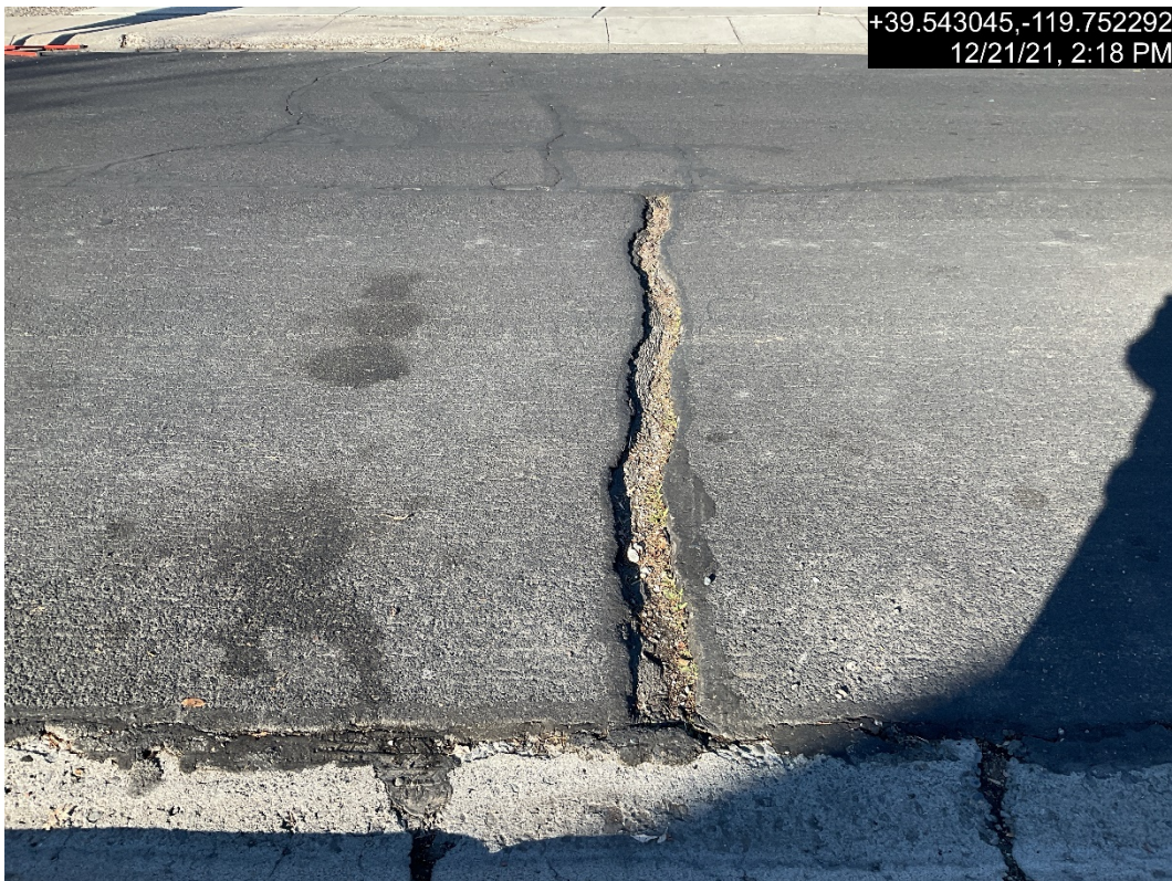
Photograph 2: Example of Wide Thermal Crack within H Street from Pyramid Way to 7 th Street
