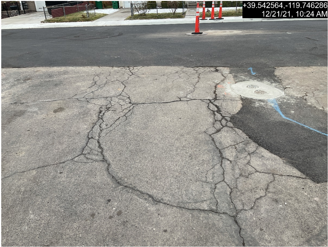
Photograph 10: Example of Fatigue cracking at G St at Interface of recent Neighborhood Streets Project
