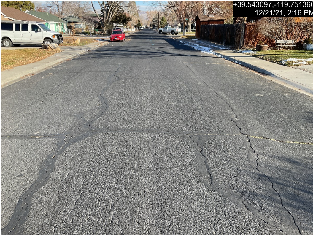
Photograph 3: Typical Pavement Condition for H Street from 7 th Street to 6 th Street
