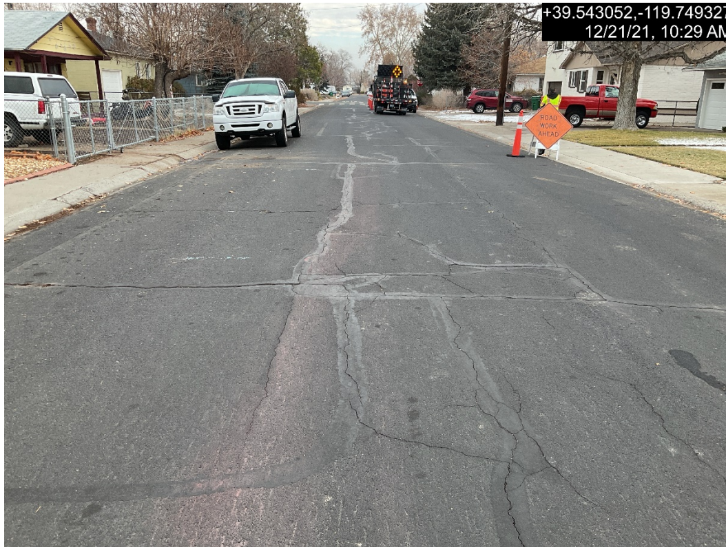
Photograph 7: Typical Pavement Condition for H Street from 5 th Street to 4 th Street
