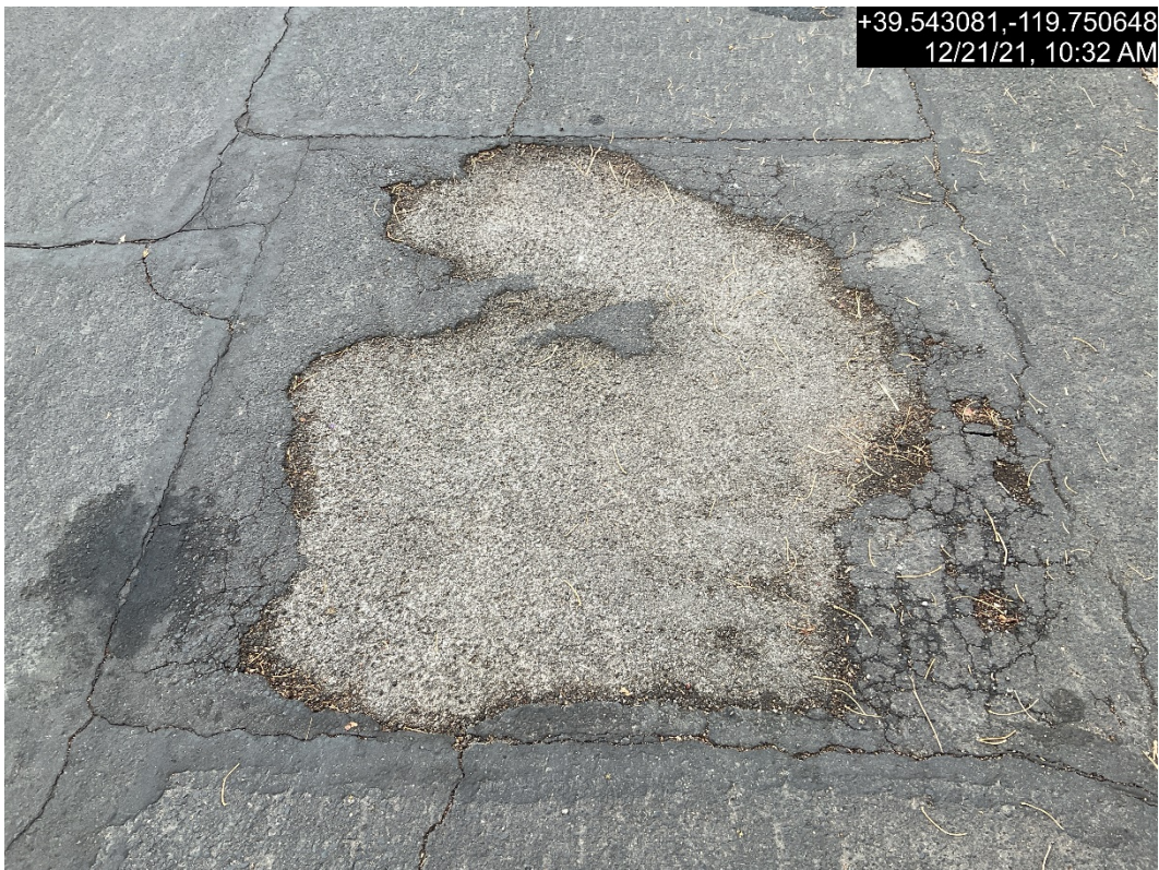
Photograph 6: Example of Localized Pothole within H Street from 6 th Street to 5 th Street
