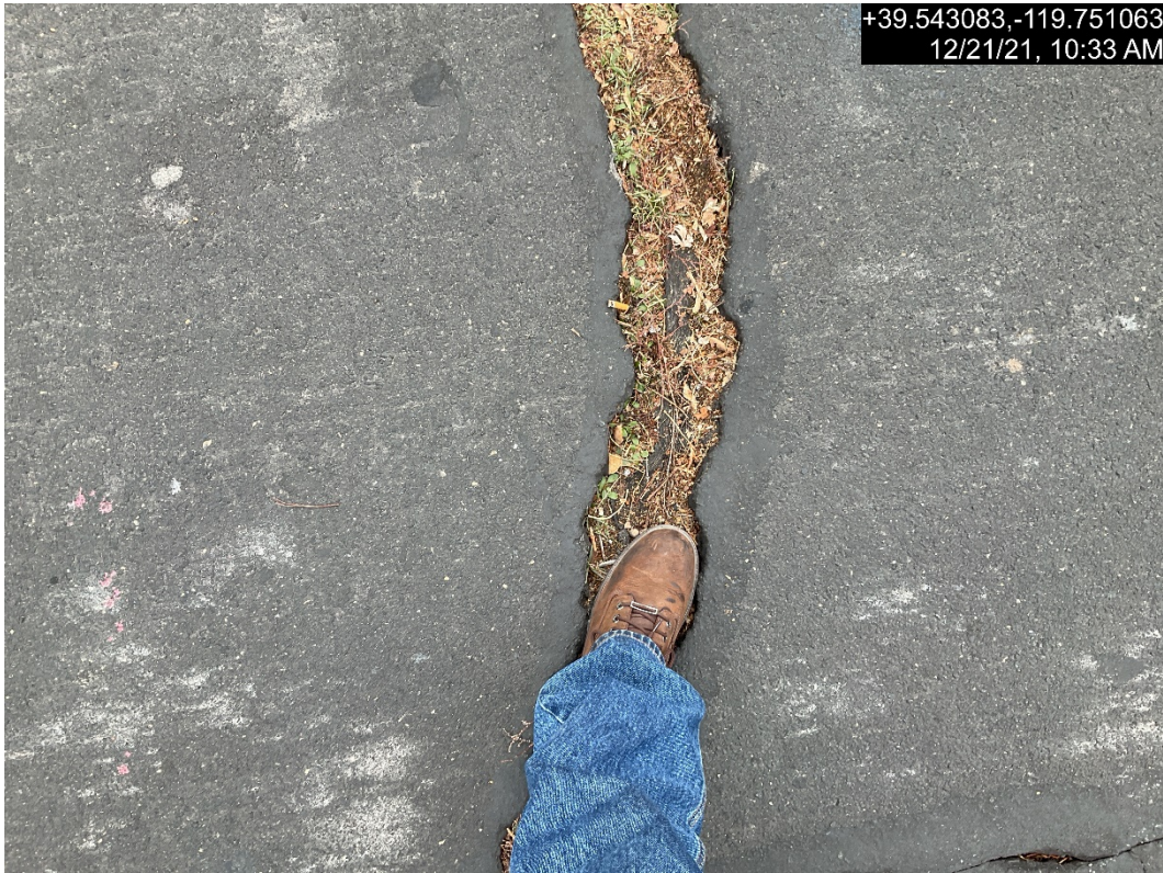
Photograph 4: Example of Very Wide Thermal Crack within H Street from 7 th Street to 6 th Street
