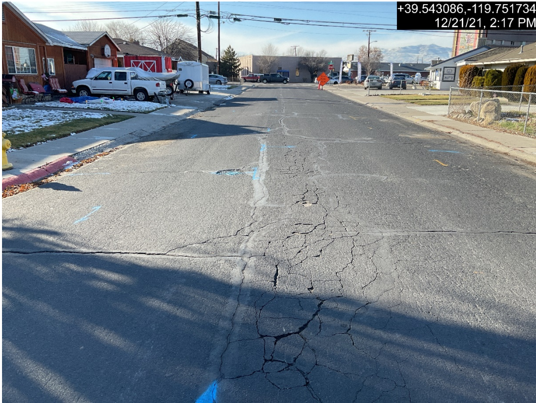
Photograph 1: Typical Pavement Condition for H Street from Pyramid Way to 7 th Street
