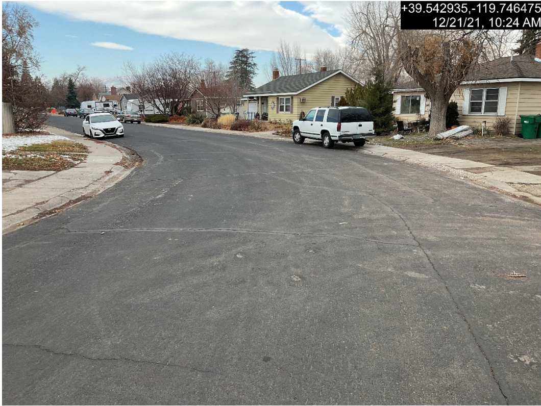
Photograph 9: Typical Pavement Condition for H Street from 4 th Street to G Street
