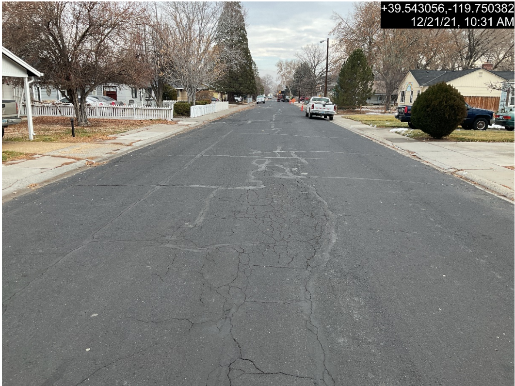
Photograph 5: Typical Pavement Condition for H Street from 6 th Street to 5 th Street
