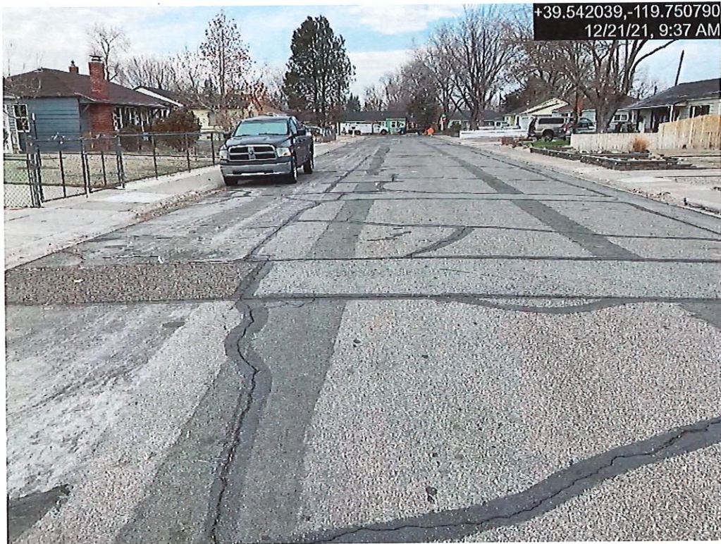
Photograph 2: Typical Pavement Condition for 6th Street from G Street to H Street
