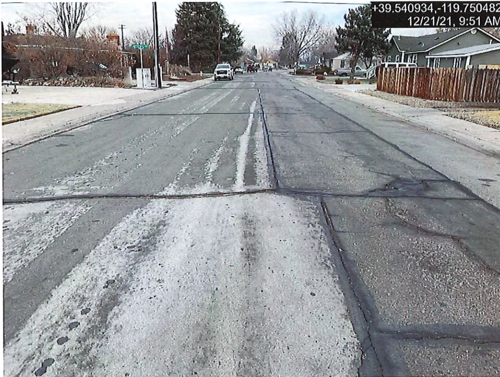
Photograph 4: Typical Pavement Condition for 6th Street from G Street to Prater Way
