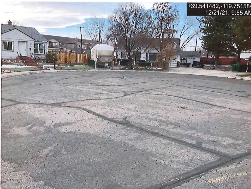
Photograph 10: Typical Pavement Condition for G Street from 6 th Street to 7 th Street at Knuckle
