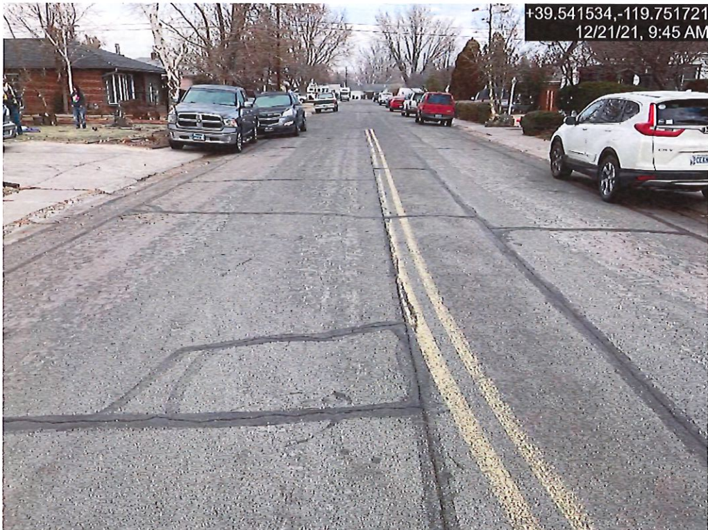
Photograph 5: Typical Pavement Condition for 7th Street from G Street to H Street
