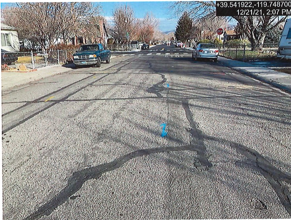
Photograph 7: Typical Pavement Condition for G Street from 4th Street to 5th Street
