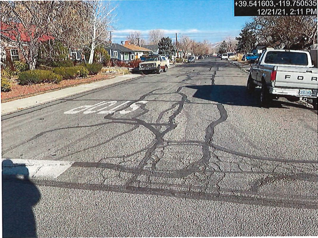
Photograph 9: Example of Fatigue Cracking on 6th Street at G Street
