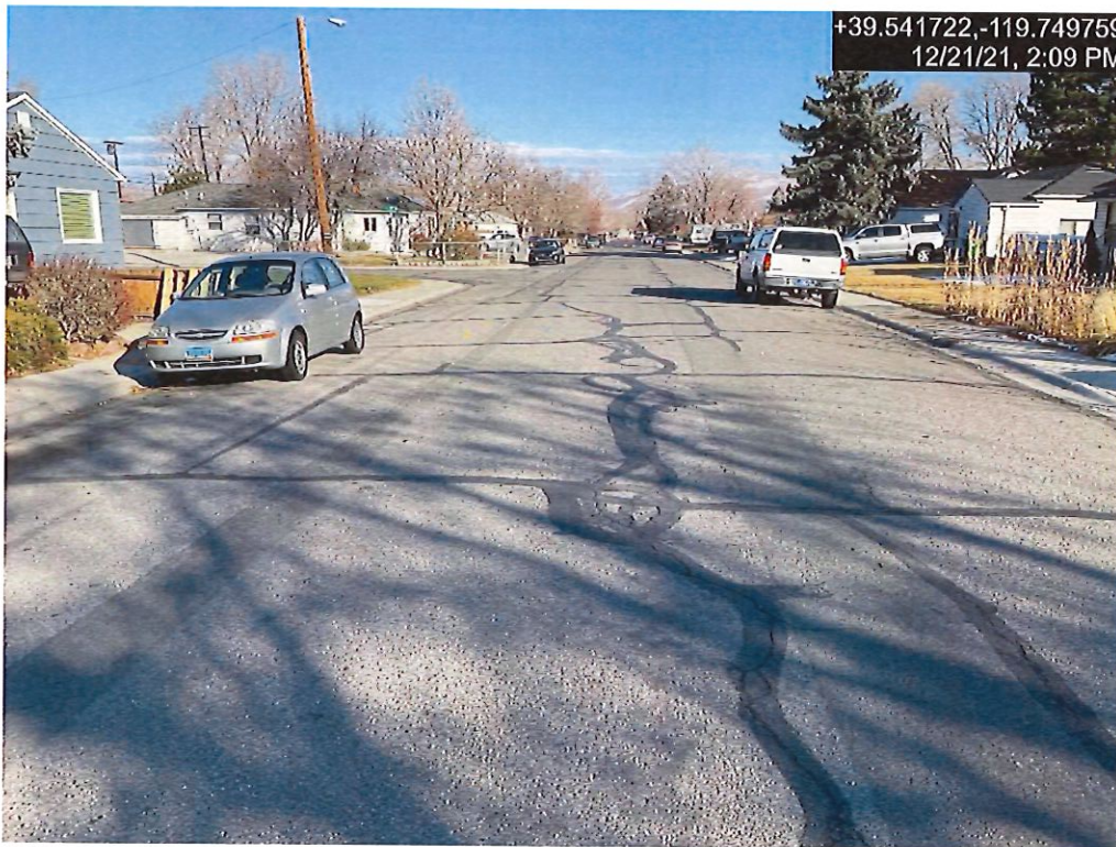
Photograph 8: Typical Pavement Condition for G Street from 5 th Street to 6 th Street
