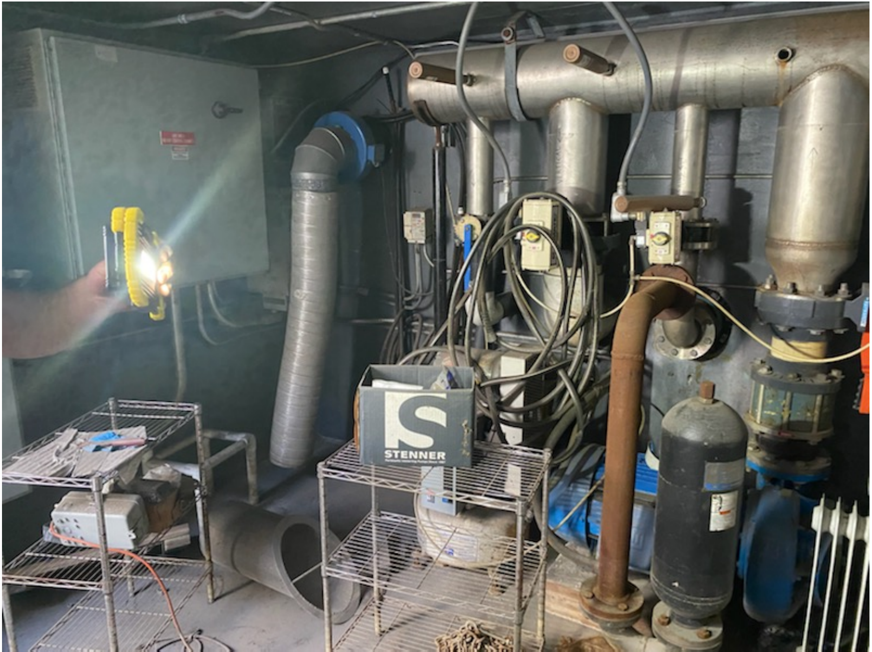
Existing Equipment Located in the Fountain Vault
