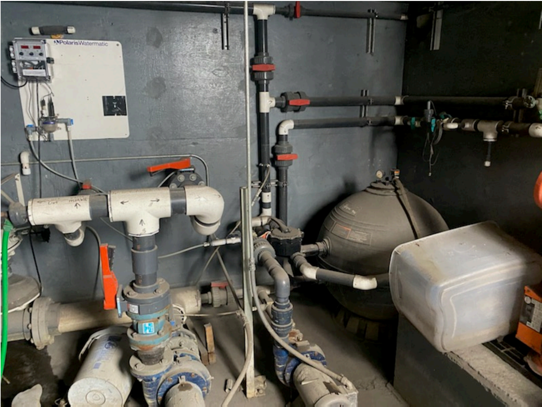
Existing Equipment Located in the Fountain Vault
