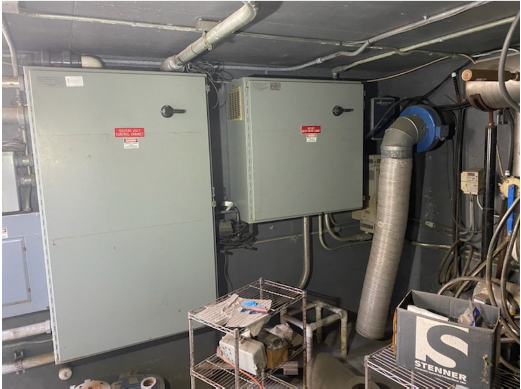
Existing Equipment Located in the Fountain Vault
