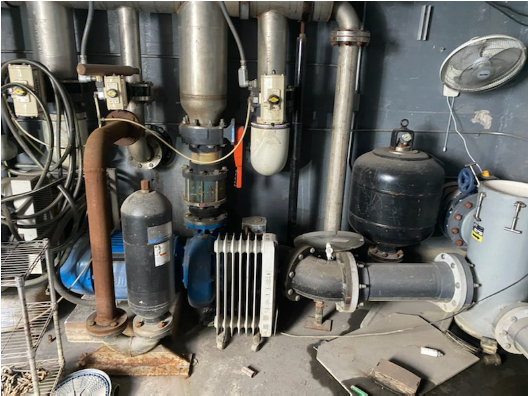
Existing Equipment Located in the Fountain Vault
